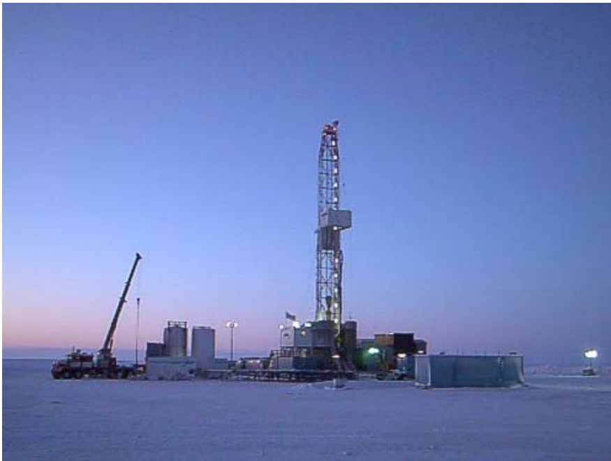
Gas Hydrate exploration, McKenzie Delta (NWT): final construction phase of drill site camp, December 2002. Photo by Hideaki Takahashi, Japex Canada Ltd.)
